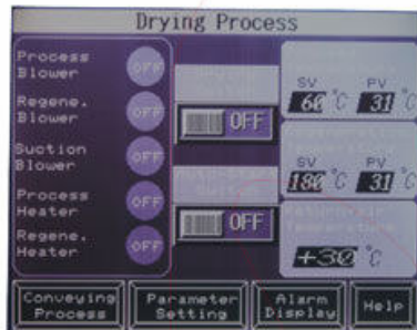
Drying process screen
